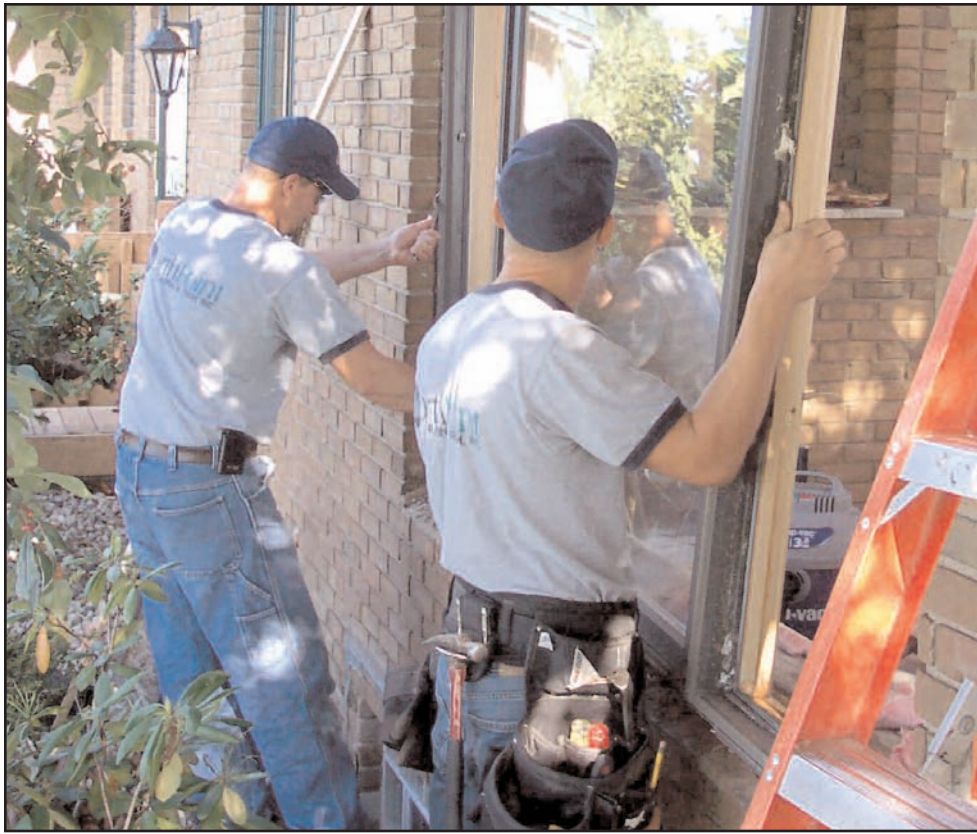
Doug Schmidt (left), co-owner of North Point Framing and Finish, helps an employee install a window. The Elmore-based company installs a variety of Andersen products.
