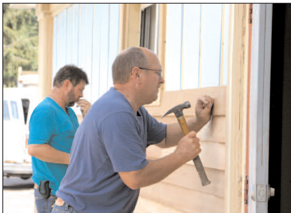
Raleigh Taylor (right) and Fred Kramer, of House Calls, nail wood siding to the renovated building at the corner of East Wayne Street and River Road in Maumee. Gianni's Italian Bistro plans to open at the location in September. MIRROR PHOTO BY SUZETTE VALENTINE
